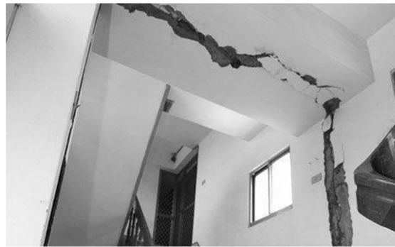
Figure 1: Cracks inside a building
